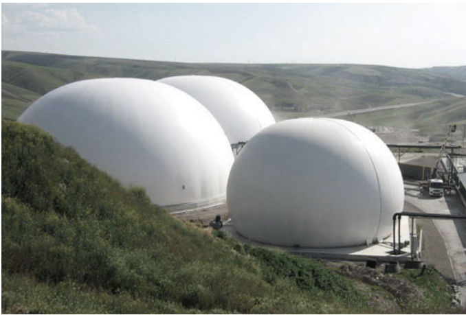
Figure 43. Methane storage a membrane holder. This kind of holder is common in contemporary large scale biogas facilities. http://www.utileengineering.co.uk/gas-holders/
