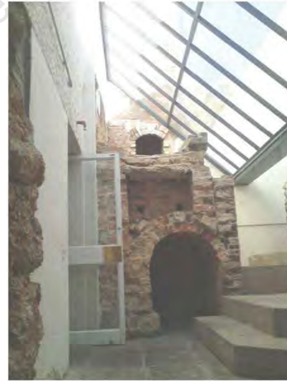
Figure 39 The bottom section of the chimney covered by a glass skylight [author 2013]
