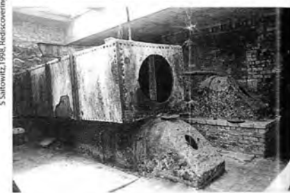
Fig. 15 A large rectangular mortar flue rests on a Coalbrookdale gas reversing valve in the basement below the tank. An air diverter valve is situated against the wall. This room filled with sand and the view from the building was dimly lit.
