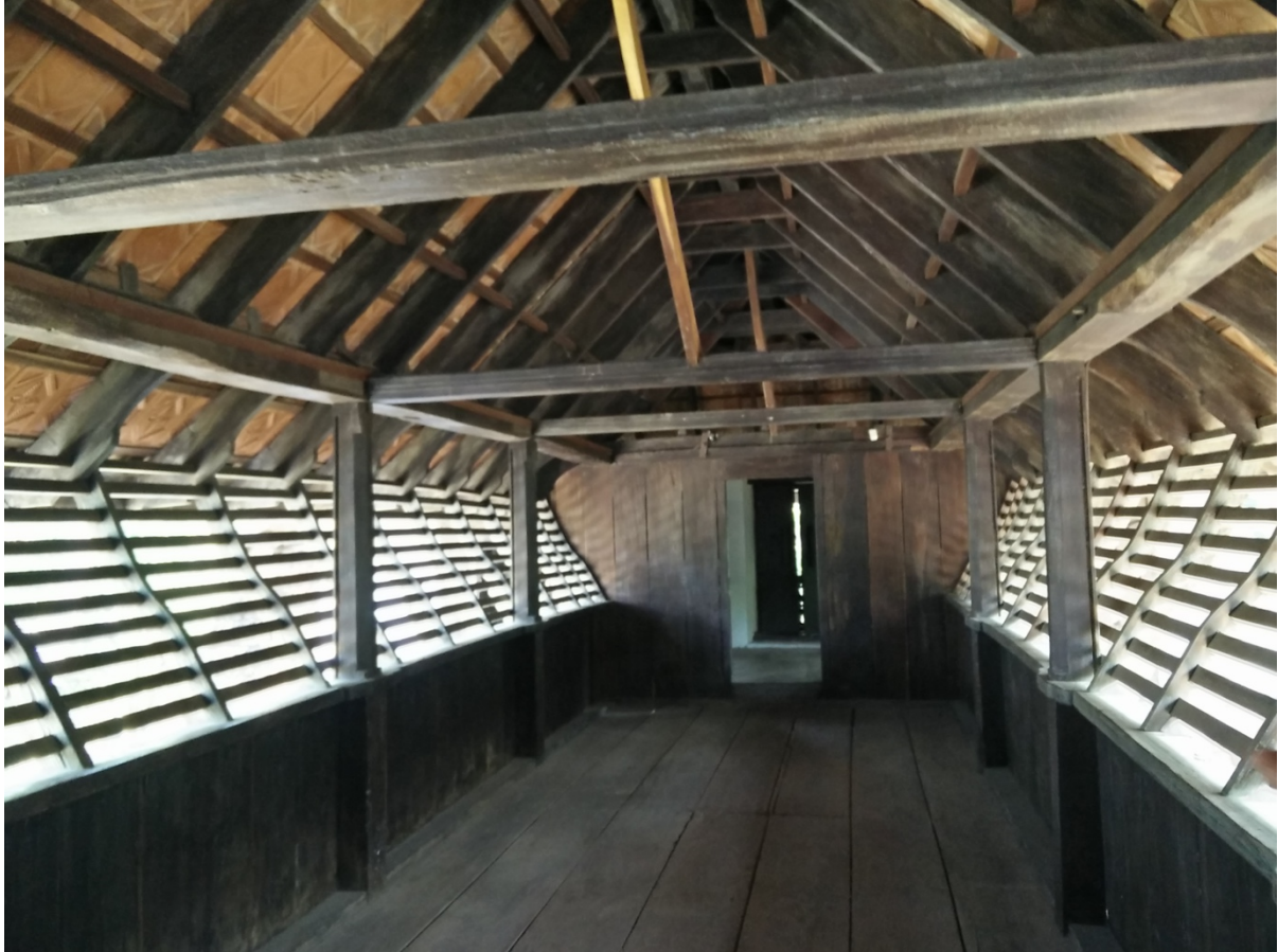
Photograph 16: Boat-like room in the upper storey of the Paravur synagogue. Photograph by Mark Aranha, January 2018.
