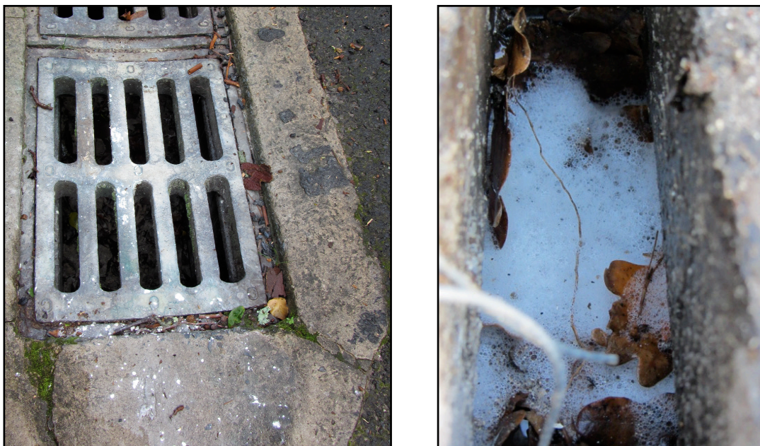
Figure 4.8: Evidence of misuse of stormwater drains. The images show evidence of wastewater containing paint (left-hand image) and detergents (right-hand image) dumped or discharged into the storm drain. Photos taken by Elizabeth Ward.
