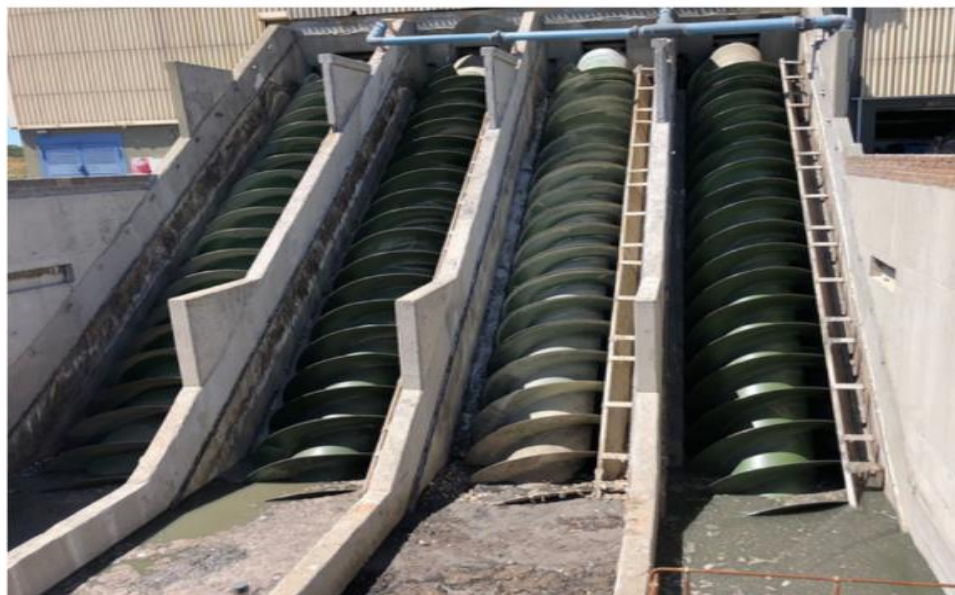
Image 5.4. Archimedes Screws at the Cape Flats Wastewater Treatment Works (CFWWTW). (Source: Independent Online, 2021).
