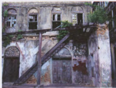
Mombasa delapidated house [Author's own]
