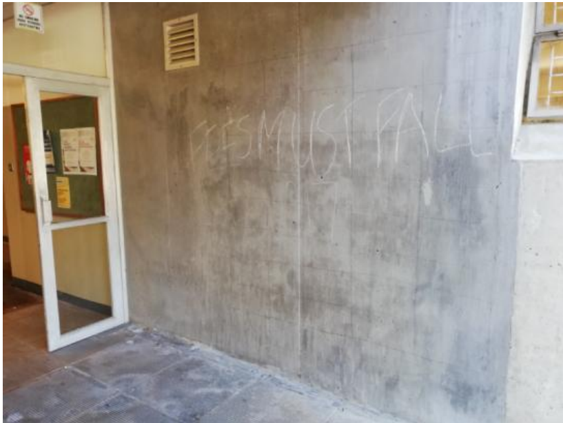
Figure 33: Location for the cover depth assessment on the ground floor of the south side of the Neville Alexander building
