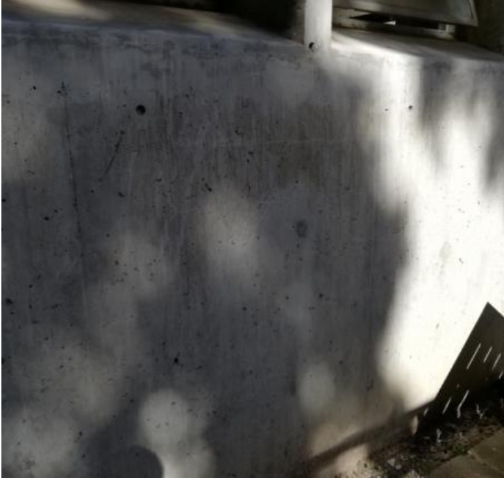
Figure 30: Location from which a core was extracted on the ground floor of the North side of the Neville Alexander building
