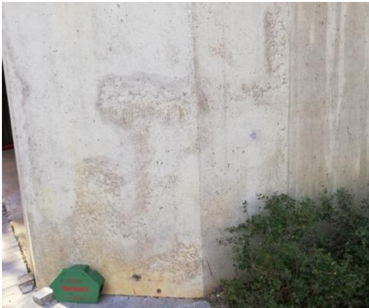
Figure 27: Location from which a core was extracted on the ground floor of the South side of the Neville Alexander building
