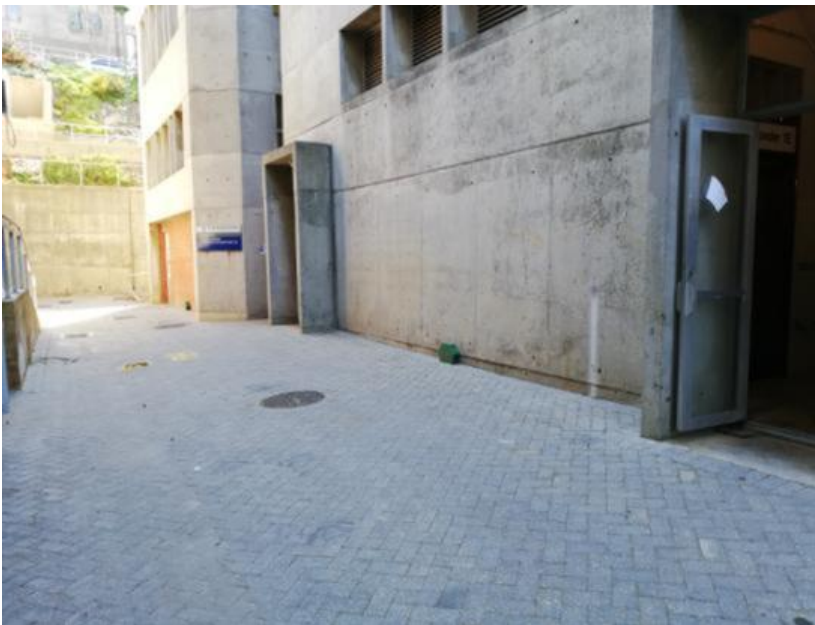
Figure 84: Location for the cover depth assessment on the ground floor of the west side of the Neville Alexander building
