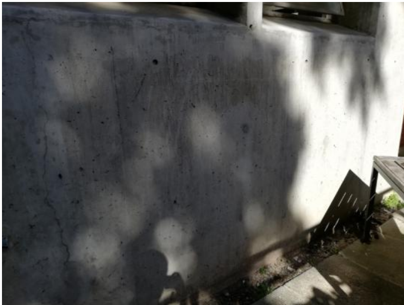
Figure 39: Location for the cover depth assessment on the ground floor of the north side of the Neville Alexander building
