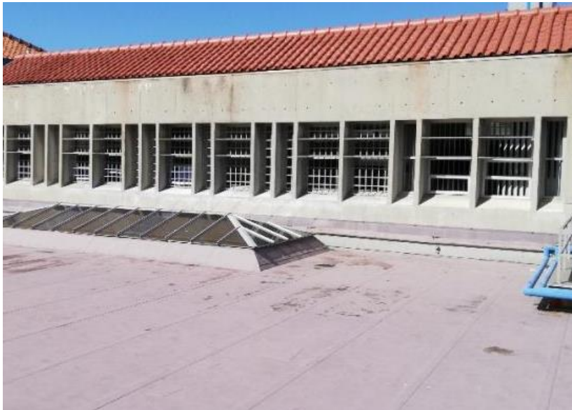
Figure 88: Location for the cover depth assessment on the 3 rd floor of the north side of the Neville Alexander building
