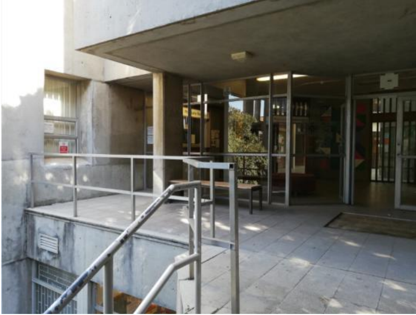
Figure 83: Location for the cover depth assessment on the 1 st floor of the east side of the Neville Alexander building zoomed out
