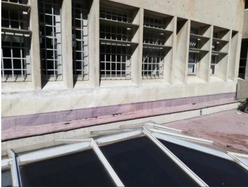
Figure 40: Location for the cover depth assessment on the 3 rd floor of the north side of the Neville Alexander building
