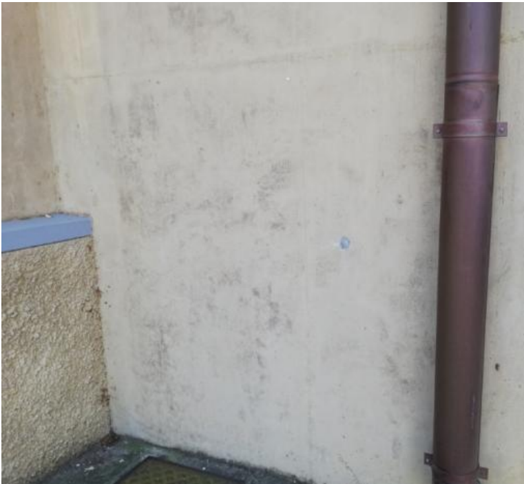
Figure 31: Location from which a core was extracted on the ground floor of the West side of the Hoerikwaggo building
