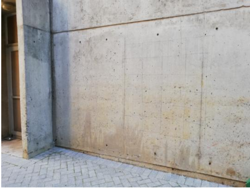
Figure 36: Location for the cover depth assessment on the ground floor of the west side of the Neville Alexander building
