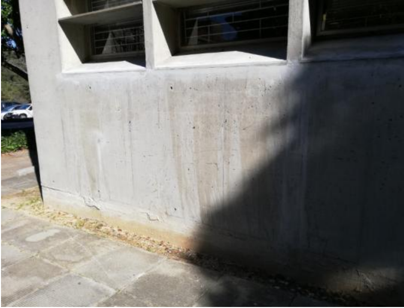
Figure 34: Location for the cover depth assessment on the ground floor of the east side of the Neville Alexander building
