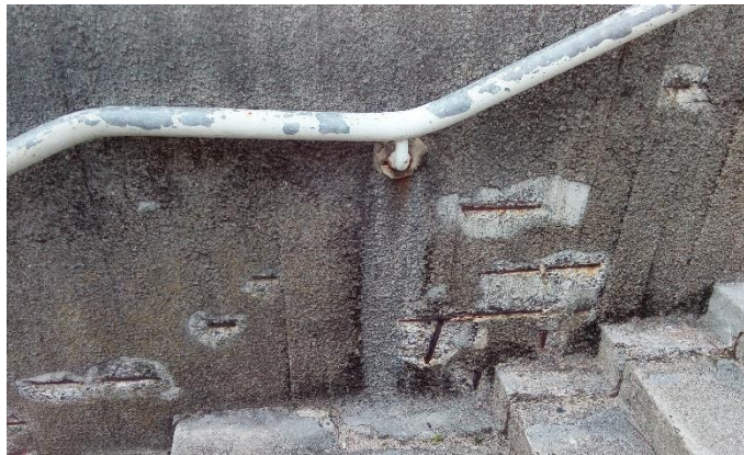
Figure 7: Concrete, which has spalled
