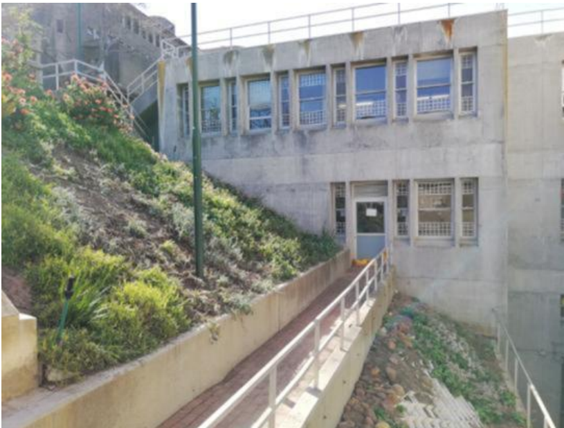
Figure 86: Location for the cover depth assessment on the 1 st floor of the west side of the Neville Alexander building
