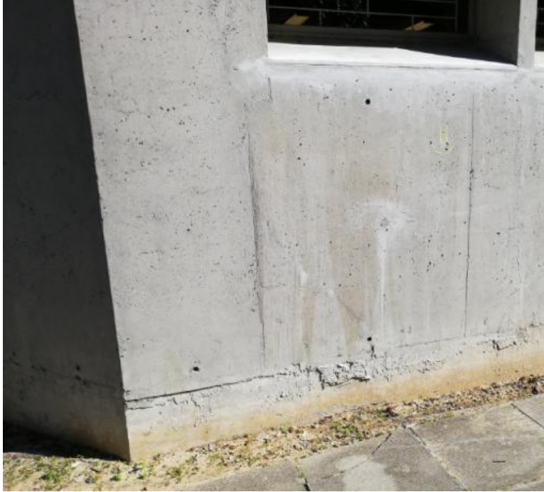
Figure 28: Location from which a core was extracted on the ground floor of the East side of the Neville Alexander building
