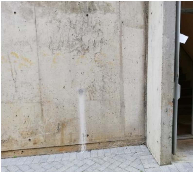
Figure 29: Location from which a core was extracted on the ground floor of the West side of the Neville Alexander building
