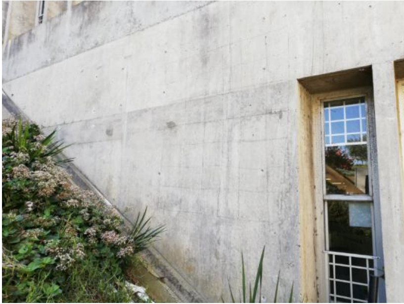
Figure 38: Location for the cover depth assessment on the 1 st floor of the west side of the Neville Alexander building
