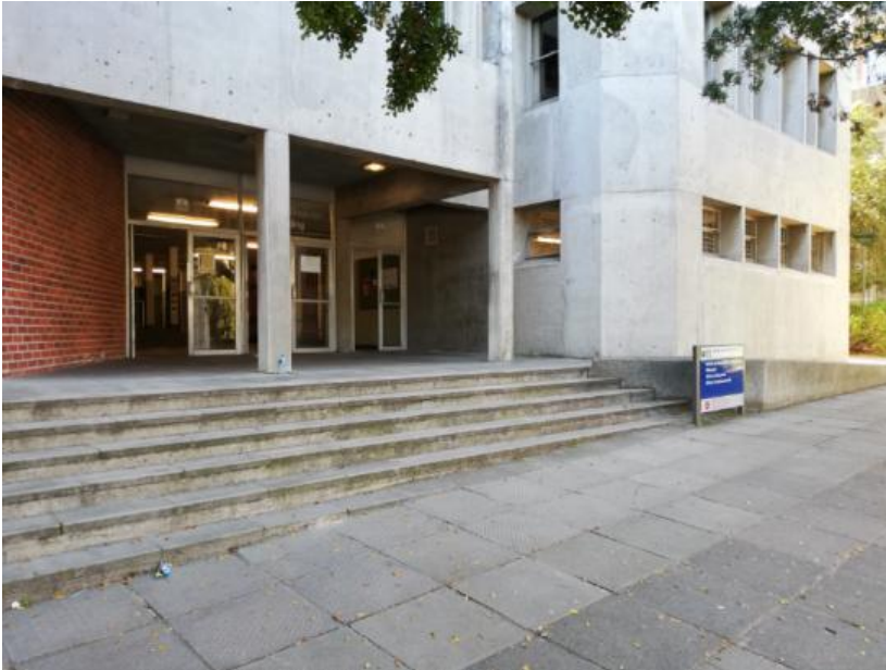
Figure 81: Location for the cover depth assessment on the ground floor of the south side of the Neville Alexander building zoomed out
