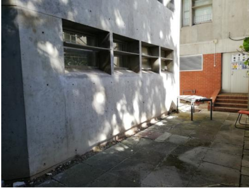
Figure 87: Location for the cover depth assessment on the ground floor of the north side of the Neville Alexander building
