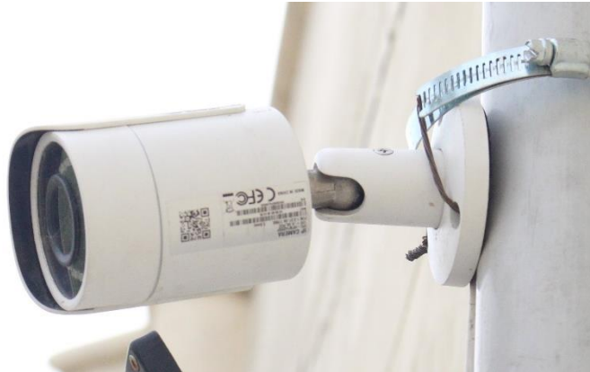
Figure 124 Dahua Network Camera
