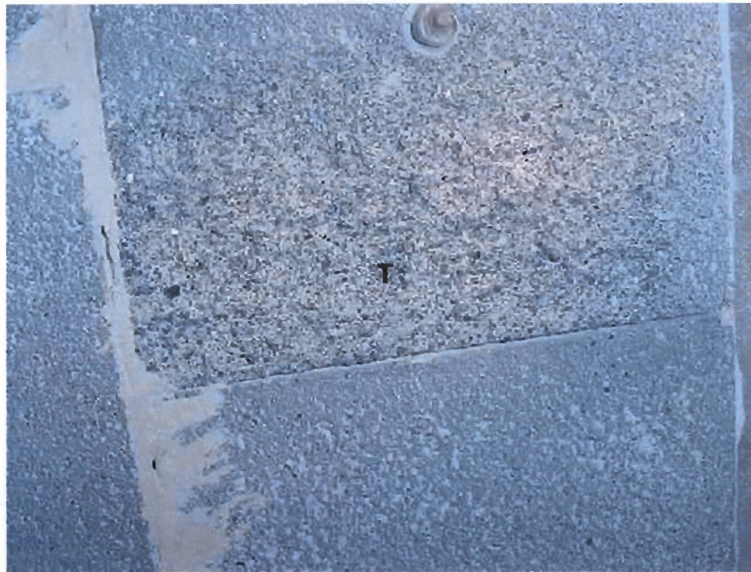
Figure 1.3: A picture showing the conditions of the SiC tiles on the Unit 6 Flue Gas Ducts at the Majuba Power Station. One tile, T, has been eroded away while adjacent tiles are still intact.
