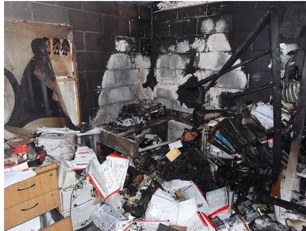
Figure 39 The Ikamva office after the bombing [Ikamva Image repository, 2011]
