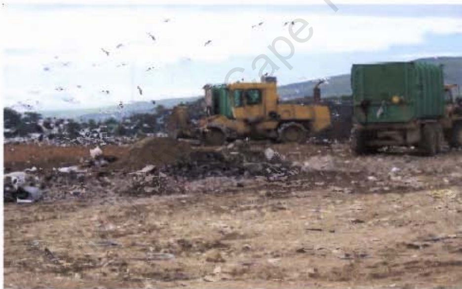
Figure 6.14 Compacting of waste and spread of daily soil cover at Vissershok landfill site
