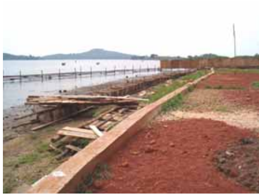
(a) Retention walls under construction after a decline in lake water levels
