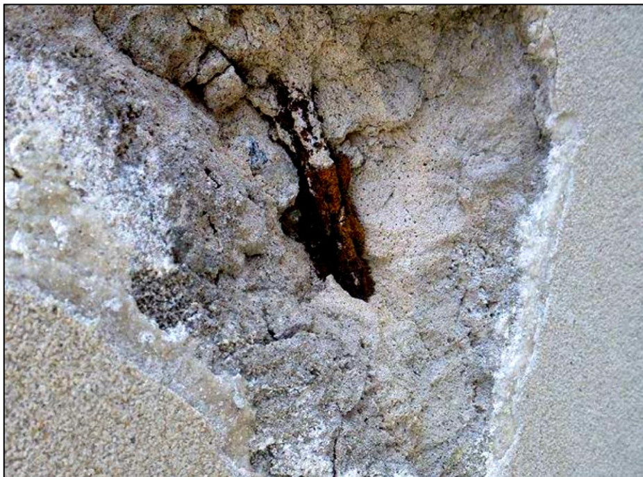
Figure 2-6: Corroded rebar and damaged concrete[33]
