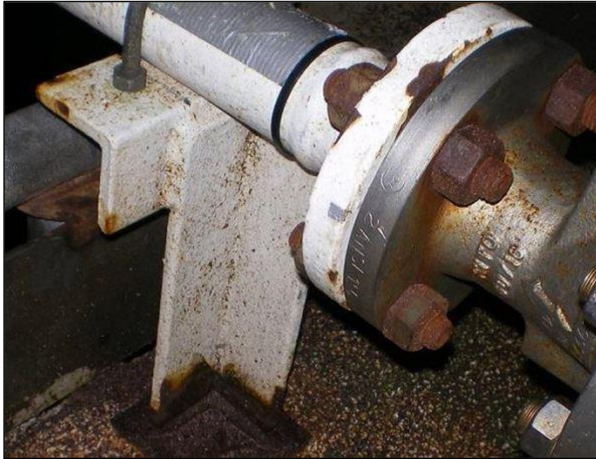
Figure 2-5: Corrosion of bolts assembling construction pipes in oil industry[16]
