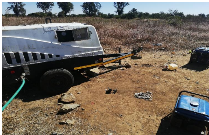
Figure 4.18: Compressor and generators (authors own)
