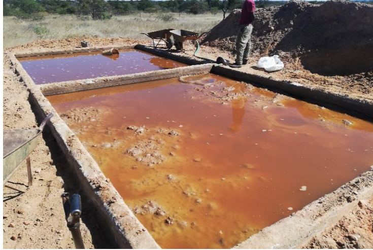
Figure 4.31: Vat Leach Tanks Site A (authors own)
