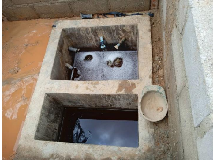
Figure 4.33: Clarifier (authors own)
