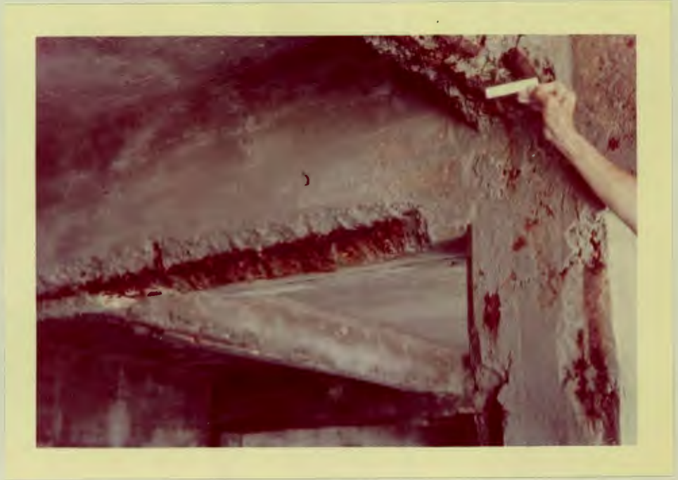
Marine corrosion at Muizenberg.
