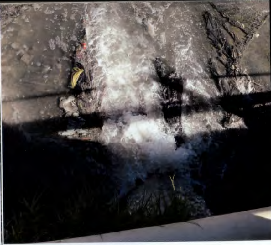
storm water entering from one of the four entrance points
