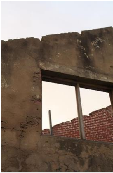
Figure 2 Abandoned building within the Whaling Station property (Liversage, 2017)
