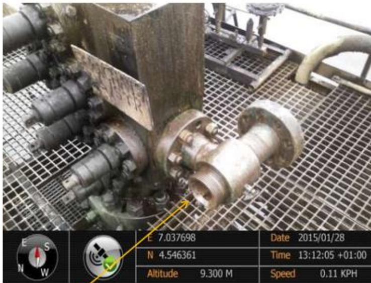
Close-up: Spill point on Cawthorne Channel1 Well9 at Captainkiri. Picture was taken during Joint Investigation of 28 th January 2015.
