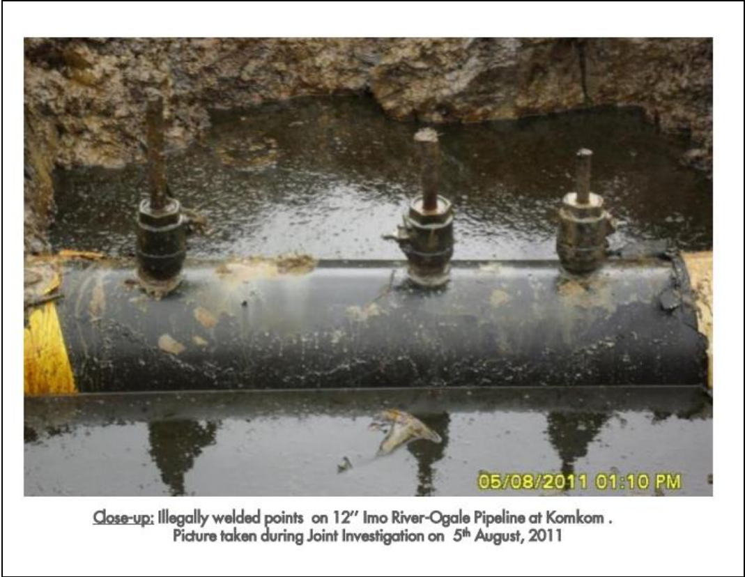
Figure 5.10 Photograph taken by the JIV showing the source of the spill. Source: Oil spill data in Nigeria http://www.shell.com.ng/sustainability/environment/oil-spills.html
