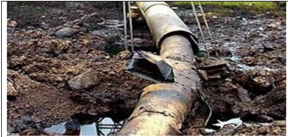
Figure 2.16 Pipeline vandalism in the Niger Delta.
