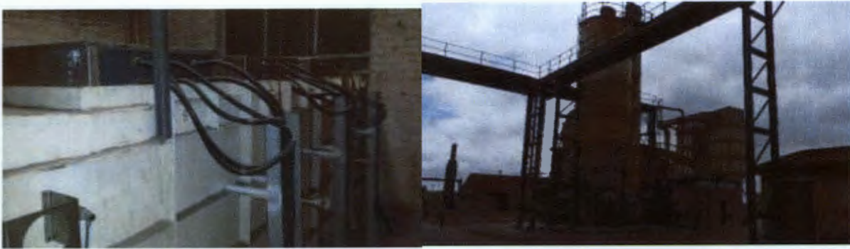
Figure 26: Atlantis Foundries electrical sand drying plant and its heat elements
