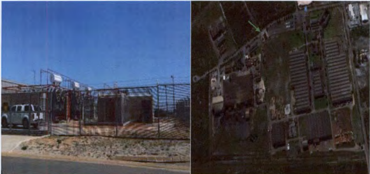
Figure 22: Atlantis Foundries main supply transformer
