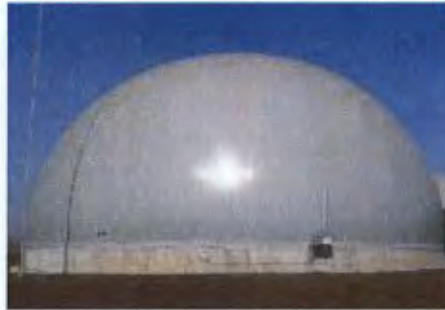
Figure 49: External double membrane gas storage
