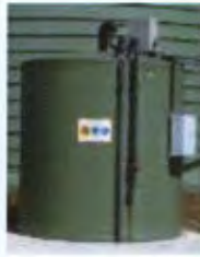
Figure 53: Ferric solution- Dosing station
