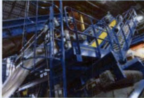
Figure 41: Example Stairways and Platforms
