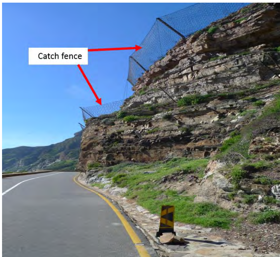
Figure 3.17: Catch fences installed along Chapman's Peak Drive to protect motorists from rock falls
