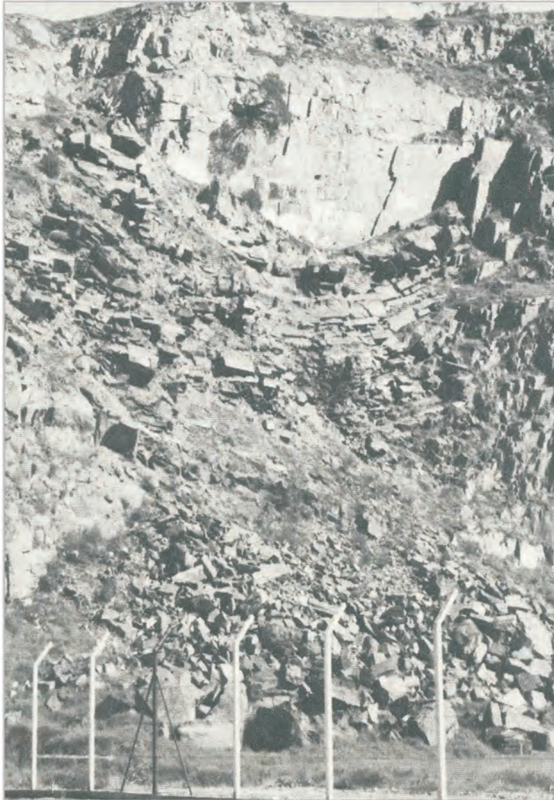
A photograph of the Strand Street Quarry showing toppling failure
