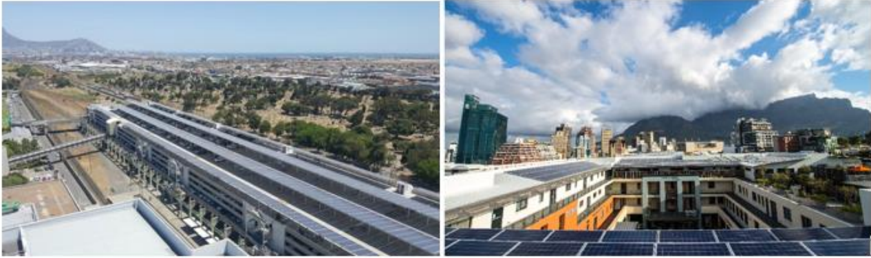
Figure 48: Ground-mount carport system at Old Mutual Park, Cape Town (left) and rooftop mounted system at Cape Quarter, Cape Town (right) (WCG, 2016) (Solar Future Energy, 2017)
