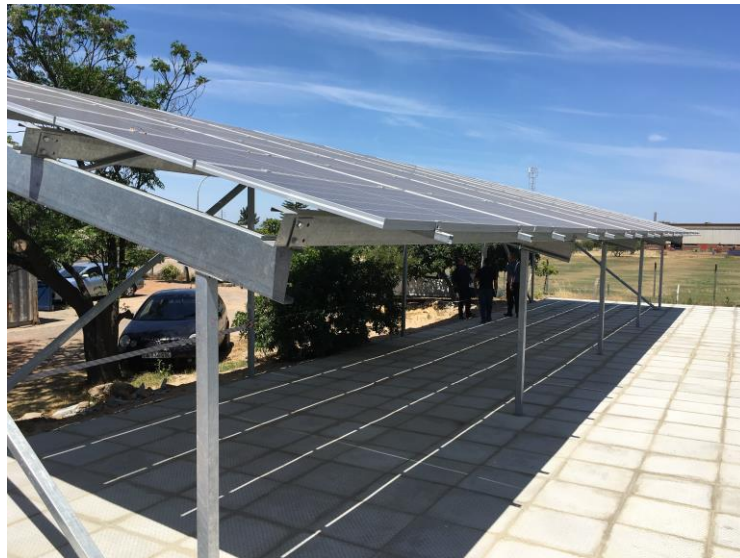
Figure 58: Completed installation of the solar photovoltaic system at Stripform Packaging
