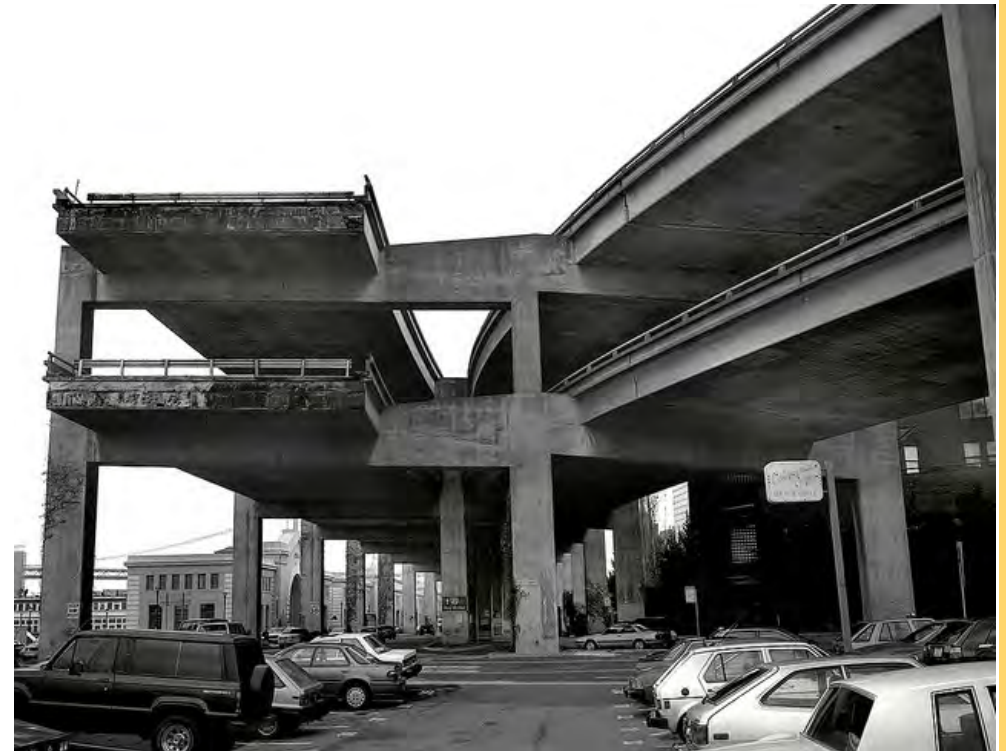
San Francisco stacked freeway after damaged by earthquake. Taken in 1990 ( www.flickr.com , 2012)
