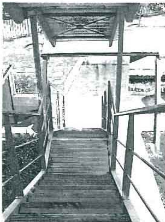
Fig. 34: New staircase outside malthouse (part of the escape route and of the visitors' circulation route)
