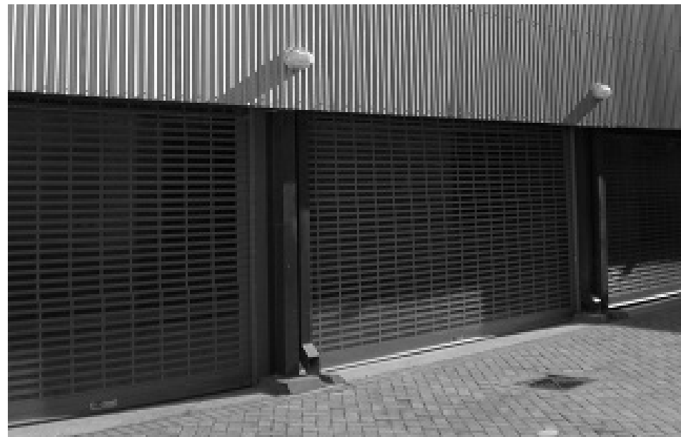
fig 70 (Aragao, 2011): Ventilated doors (closed)
