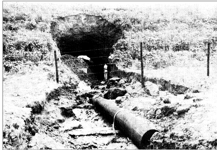
Figure 2-6, A damaged embankment constructed of dispersive soil (Source: Edgar, 1991)
