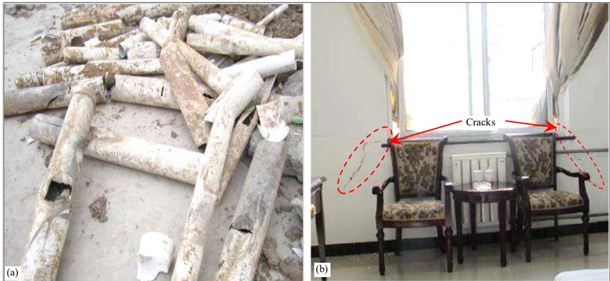
Figure 2-27, Hydrocollapse settlement triggered by heavy rainfall: (a) ruptured water pipes and (b) cracks below the window (Source: Yuan-xun et al., 2013)
