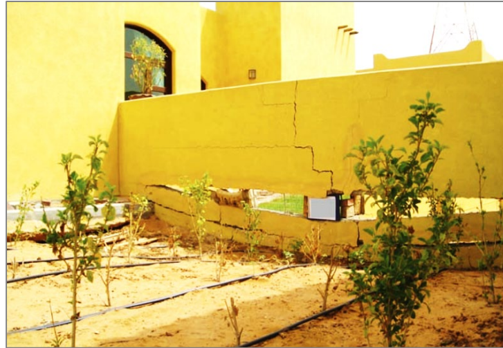
Figure 2-8, Damage on boundary wall as a result of settlement induced by collapsible soils in Abu Dhabi (Source: Vandanapu et al., 2016)
