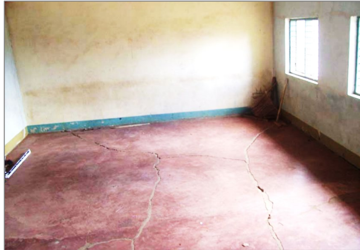
Figure 2-3, Concrete floor crack caused by expansive soil in Tanzania (Source: Lucian, 2006)
