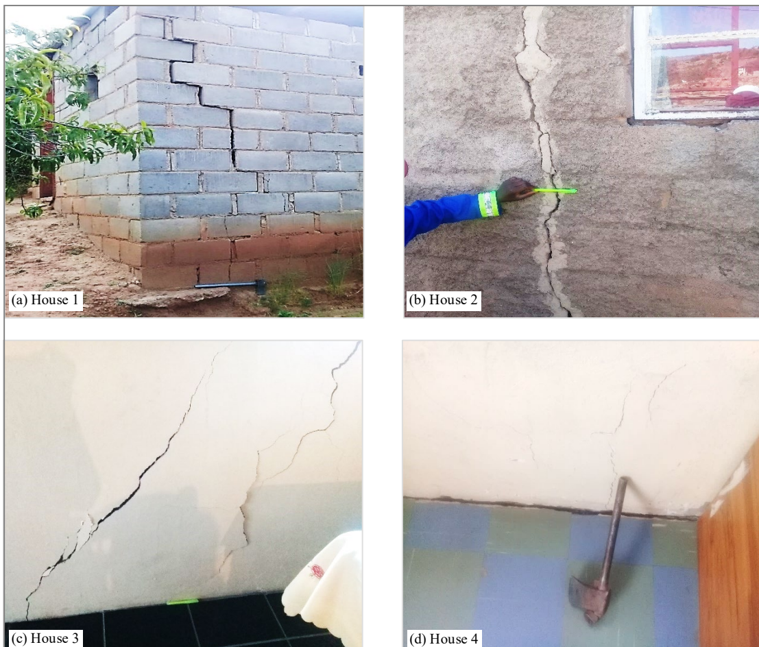
Figure 1-1, Cracks on some of the selected houses in the Mount Moorosi village
