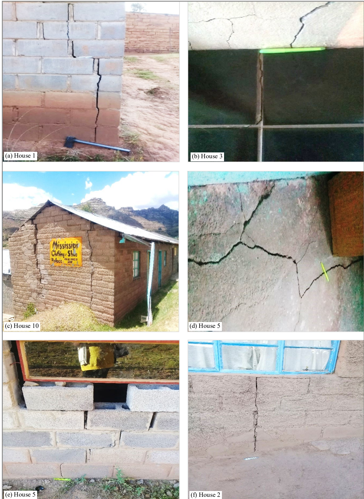
Figure 3-11, Cracks on some of the selected houses in the Mount Moorosi village
