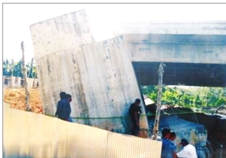
Figure 2-4, A tilted bridge abutment in Indonesia (Source: Rahardjo, 2014)
