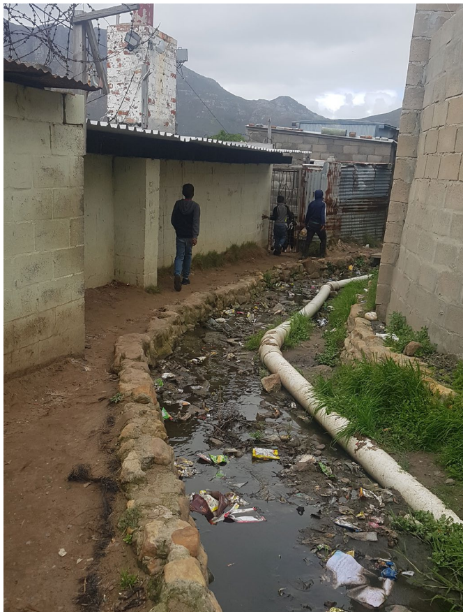
Figure 2.10: Illegal sewage connections (Source: author)
