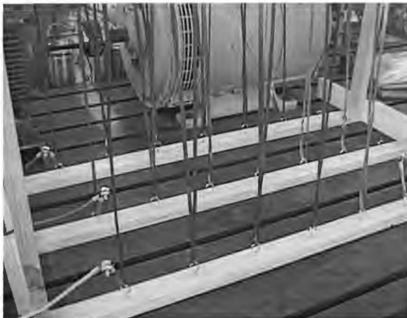
Figure 5.6 Close-up of frame and connections of constructed resistors
