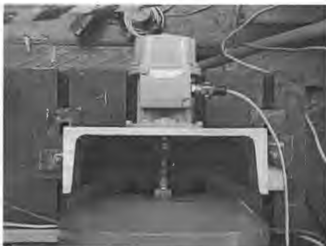
Figure 13.20 The motor shaft is extended, as shown, to allow for connection of the tachogenerator. Connection is made via a flexible coupling, to allow for misalignment, consisting of a short piece of garden hose and two jubilee clamps.
