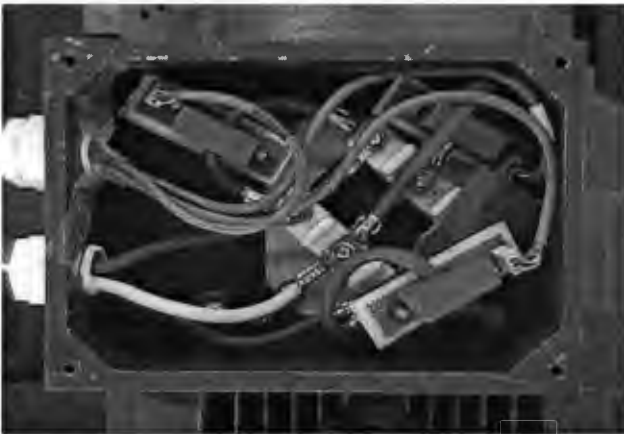
Figure 13.6 The LEM current transducers are mounted inside the terminal box, housed on top of the motor, in order to sense the individual phase currents.
