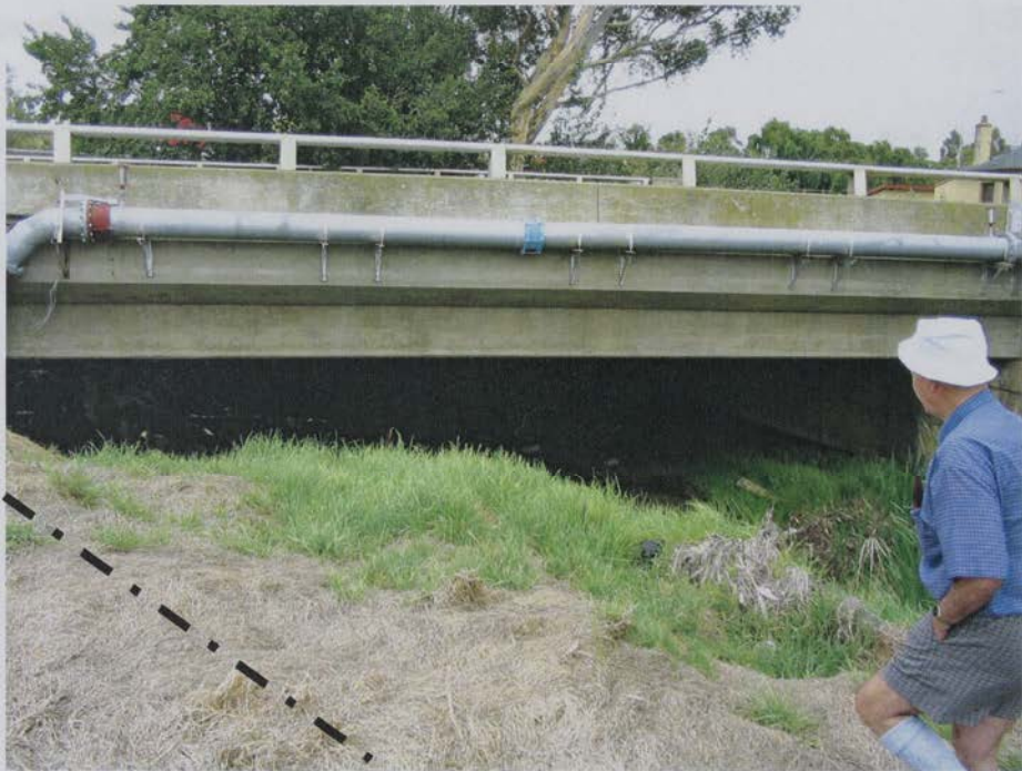
Figure 5.5: A build-up of debris underneath 'The Old Bridge' in Caledon
