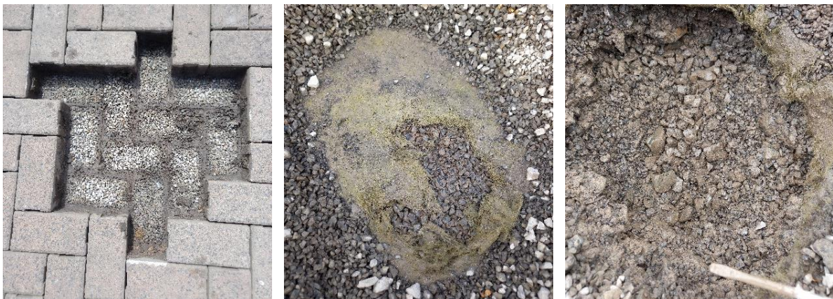
(a) Sediment outline (b) Damaged geotextile (c) Muddy film aggregates
