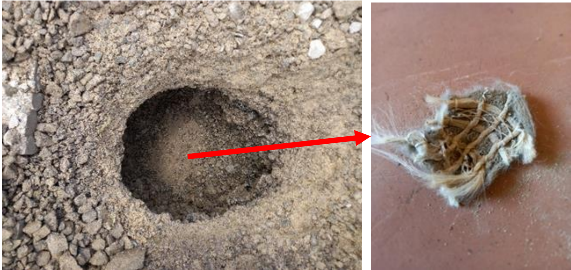
Figure E-6: Damaged bottom geotextile
