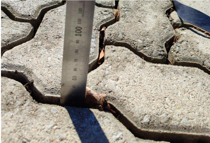
Figure 4-66: BRT-7-03 missing gritstone (up to 30 mm)
