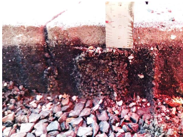
Figure E-1: Type I clogging (in the joints)
