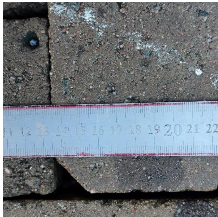
Figure 4-96: Compromised paver 'lock-up'
