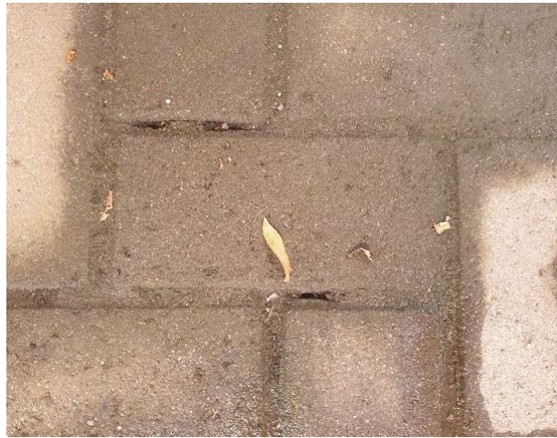
Figure 4-74: Typical sediment accumulation in joints adjacent to vegetated areas
