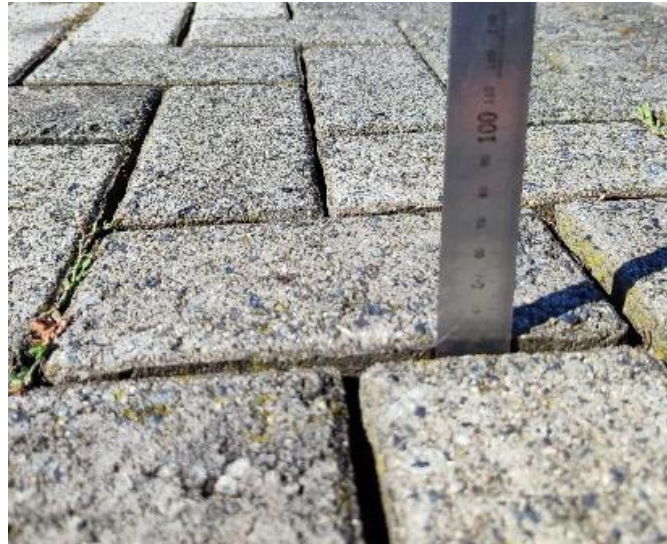
Figure 4-85: Typical PICP section with missing grit
