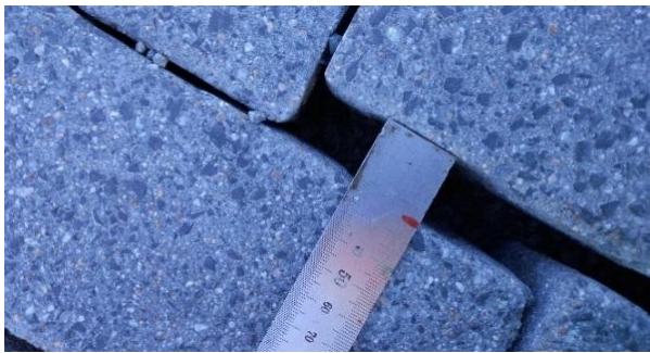
(a) Widened joints with no grid
