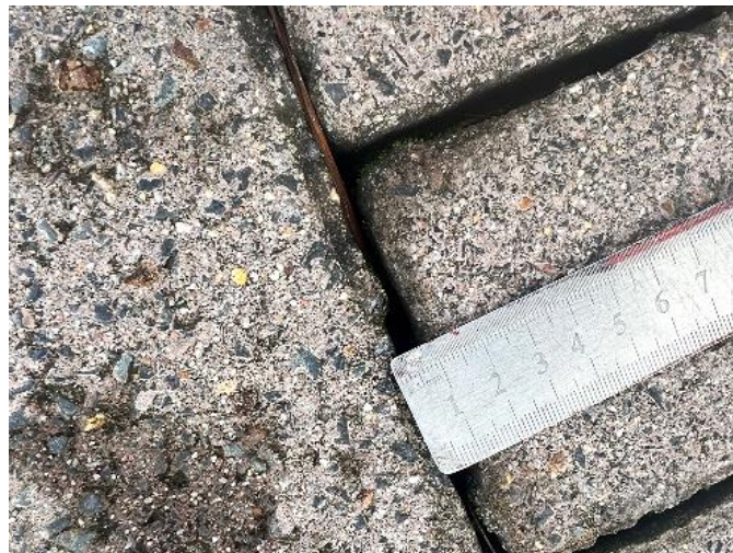
Figure 4-25: Typical PICP section with missing grit and fine sediment on the pavers
