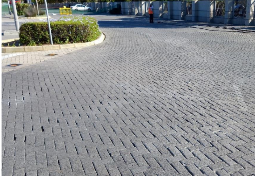
Figure 6-8: A failed PICP edge restraint at a bend in the road
