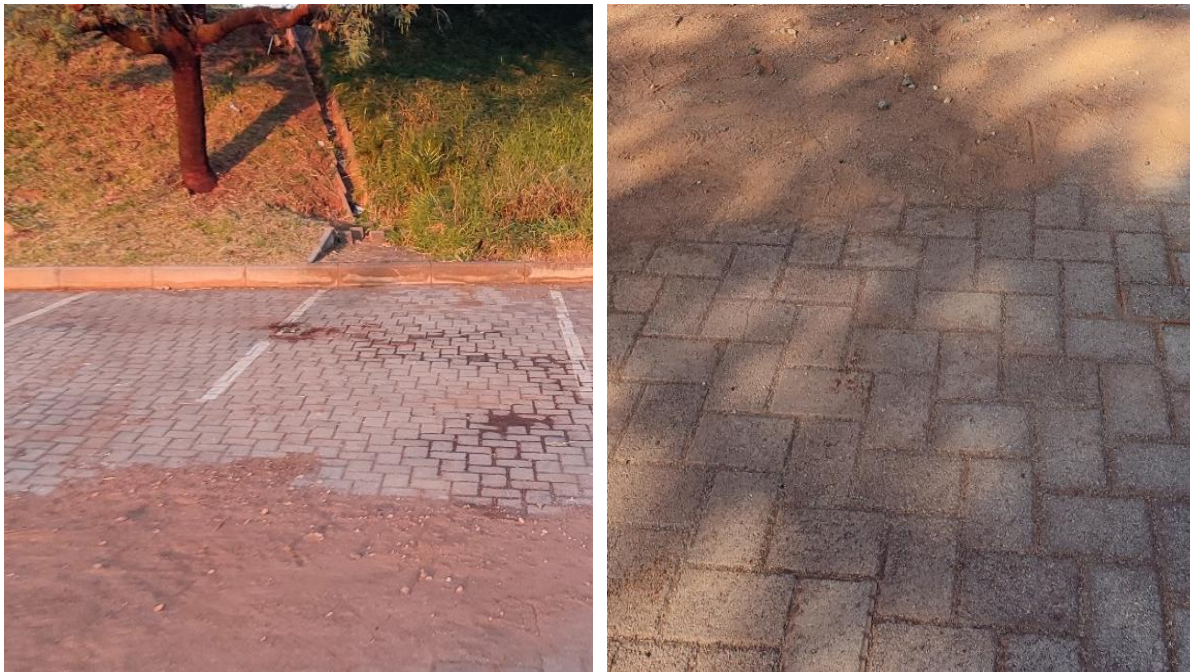
(a) Exposed sediment on a slope
