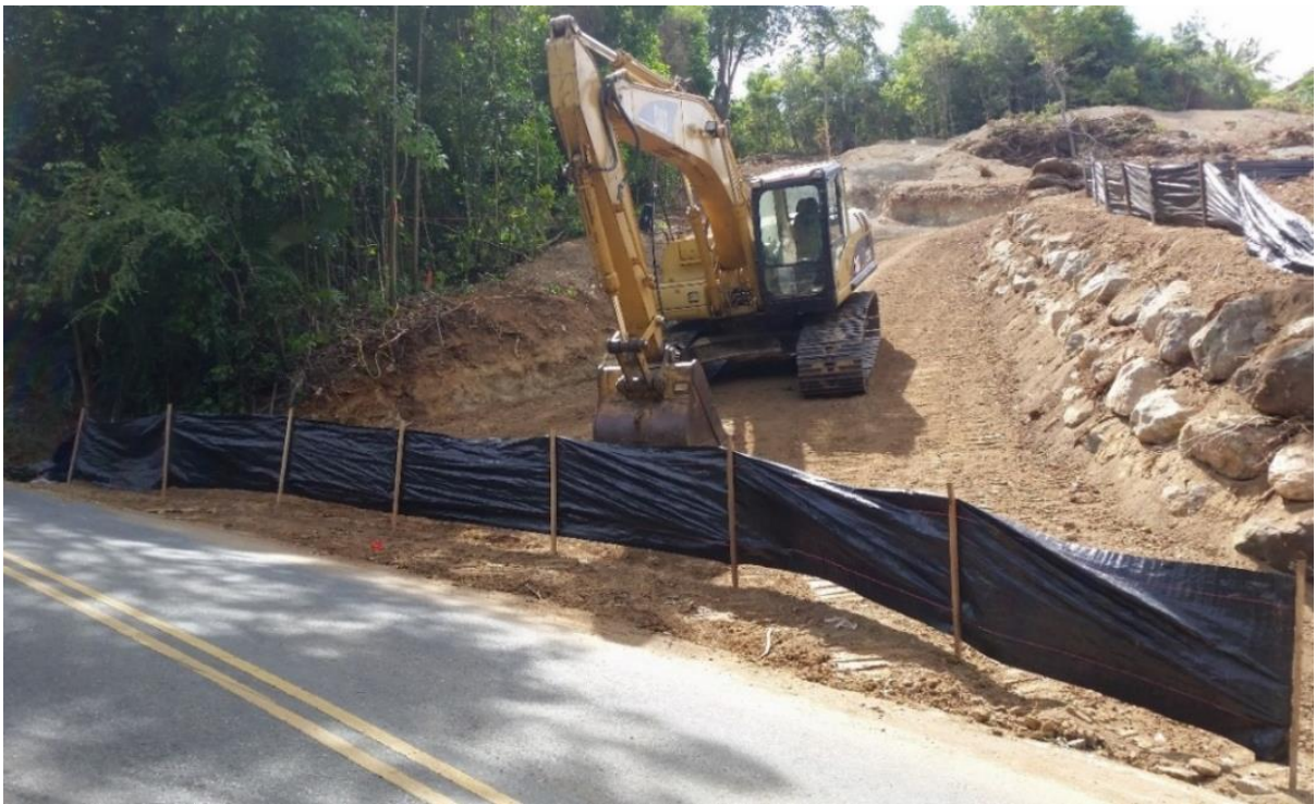
Figure 2-20: Inadequate sediment trap installation (St John Source, 2022)
