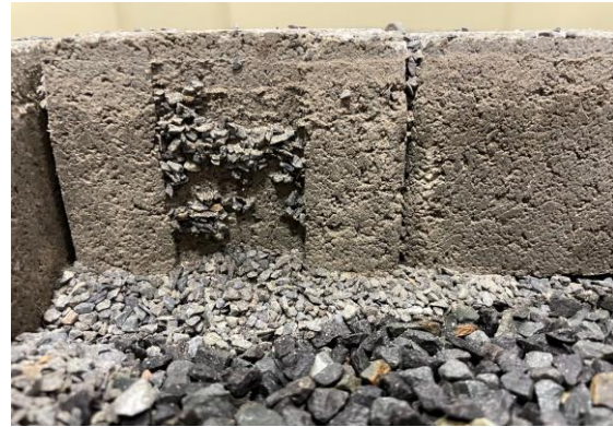
(b) Sediment in joints
