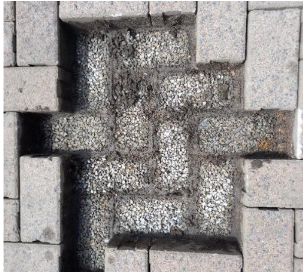
Figure E-2: Type II clogging (below the joints)
