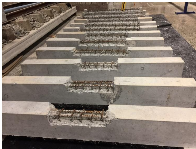
Figure 4.6 Exposed RC beam after removal of damaged cover concrete in the tension region
