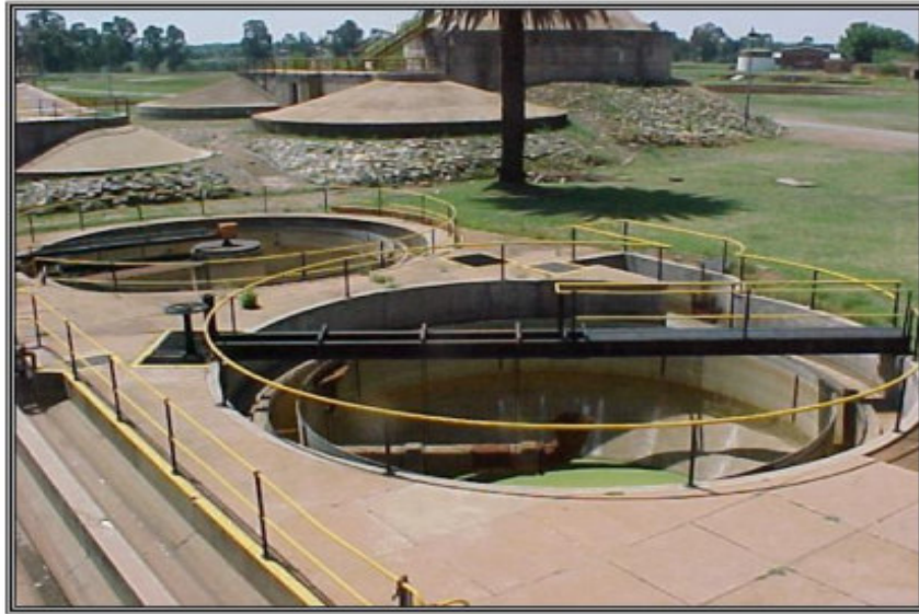
Figure 2.6: The 2 ML/d Recycling Sludge Bed Reactor (RSBR) in the BioSURE ® sewage sludge solubilisation technical-scale plant constructed at ERWAT's Ancor Works in Springs, Gauteng, South Africa.
