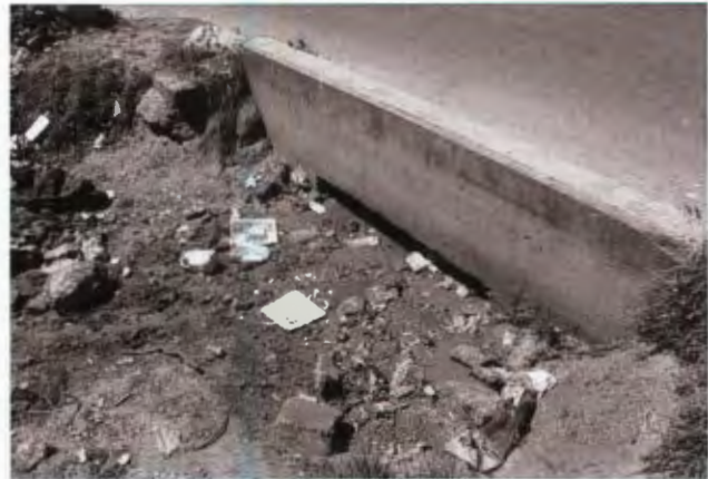
Figure 55 : Silt and rubbish accumulation in drain (Bouchard et al., 2007)
