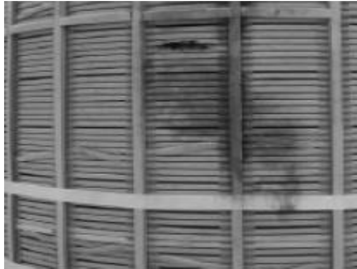
Figure 2-2: Damaged HV winding due to GICs at the Ruacana power station [Gaunt & Coetzee, 2007]
