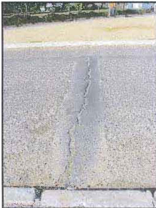
Movement at joint causing cracking in asphalt overlay. PLATE 8
