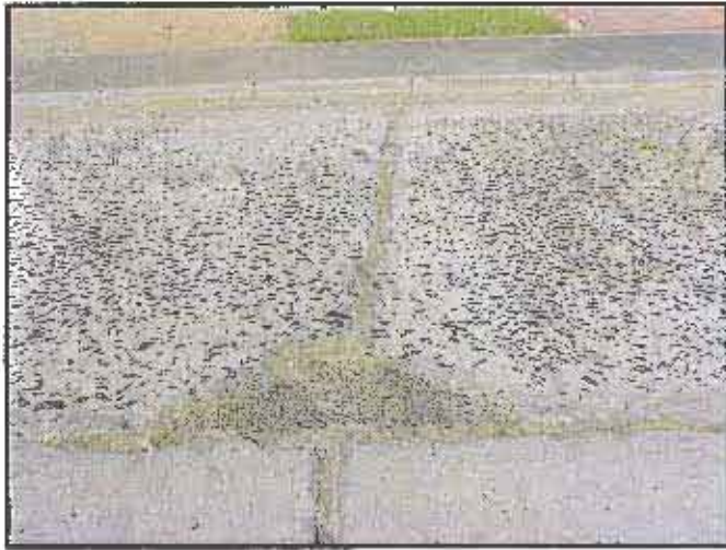
Loss of support resulting in cracking of slab corners PLATE 2
