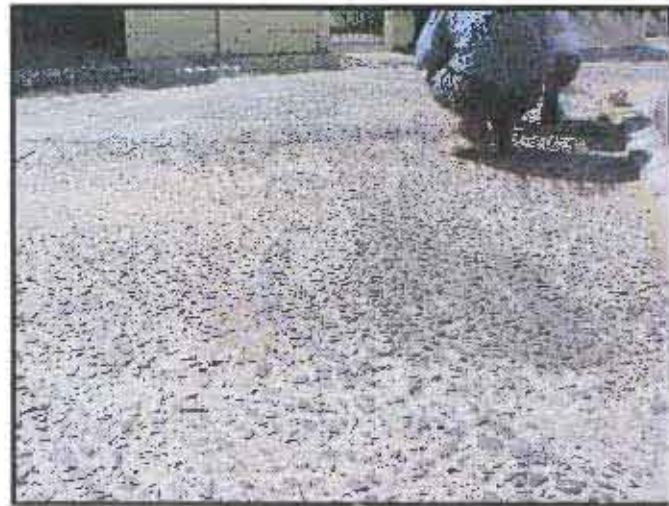
Ravelling resulting in exposed aggregate. PLATE 7
