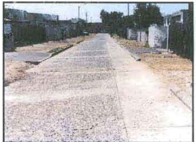
Various defects -- exposed aggregate, loss of support, joint disintegration PLATE 9
