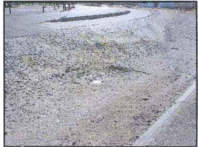
Lack of support, raveling and joint disintegration. PLATE 3
