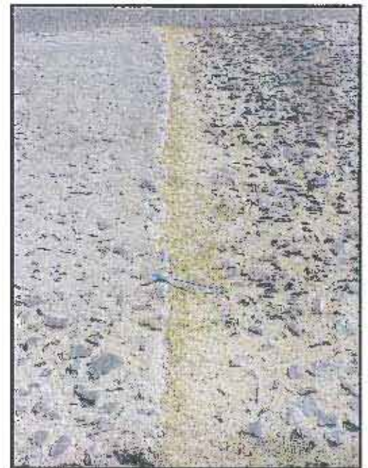
Slab faulting and exposed aggregate. PLATE 5
