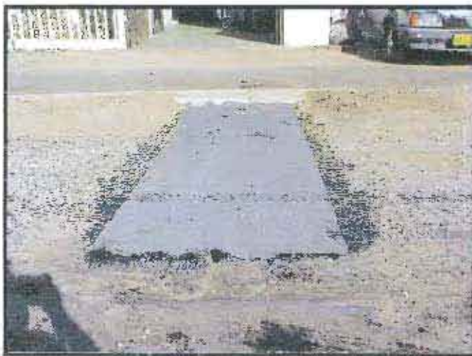
Geofabric bandage over crack. PLATE 12
