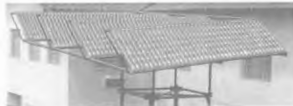
The solar water system used for a hotel in Curitiba
