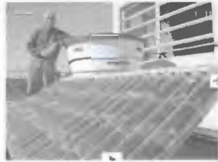
Solar water heater
