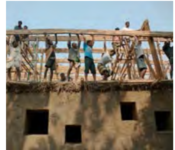
Fig 3.10: DESI centre under construction - Clay bricks for ground floor and bamboo for the first floor
