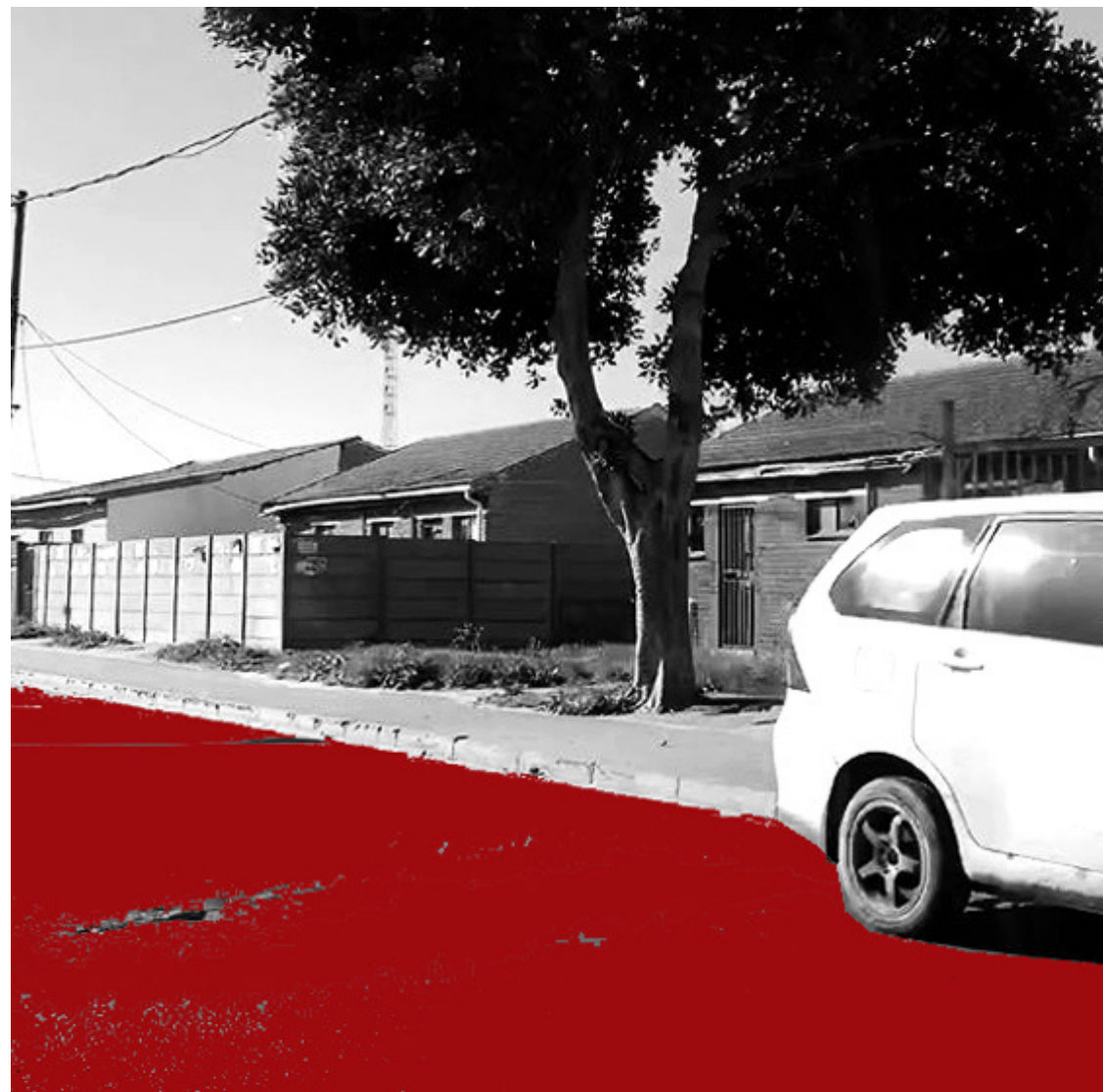
Figure 4.3.3.2d: Potholes on New Eisleben Road (Author's own, August 2022)
