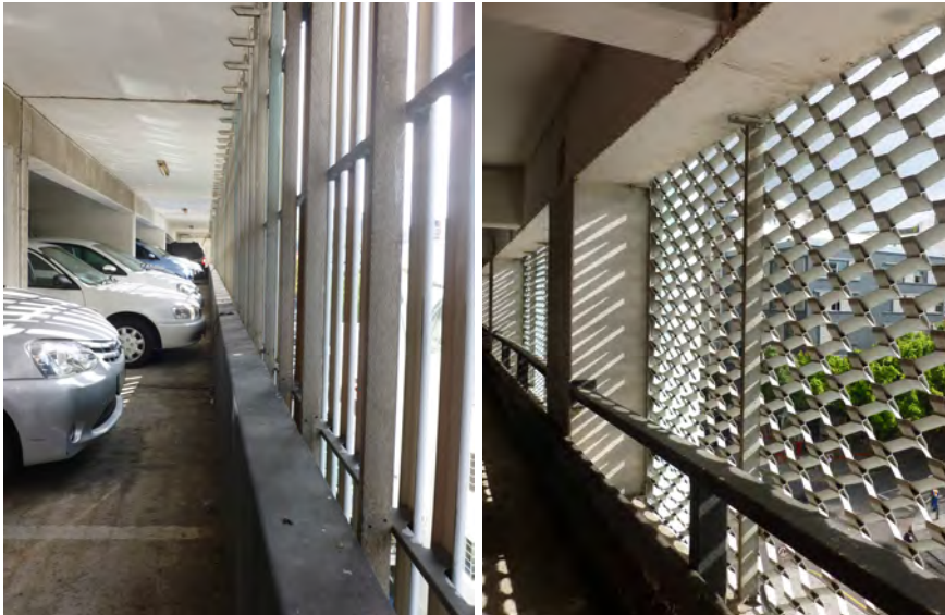
Figure 78: Images of the existing downstand conditions and screening used in the parking floors
