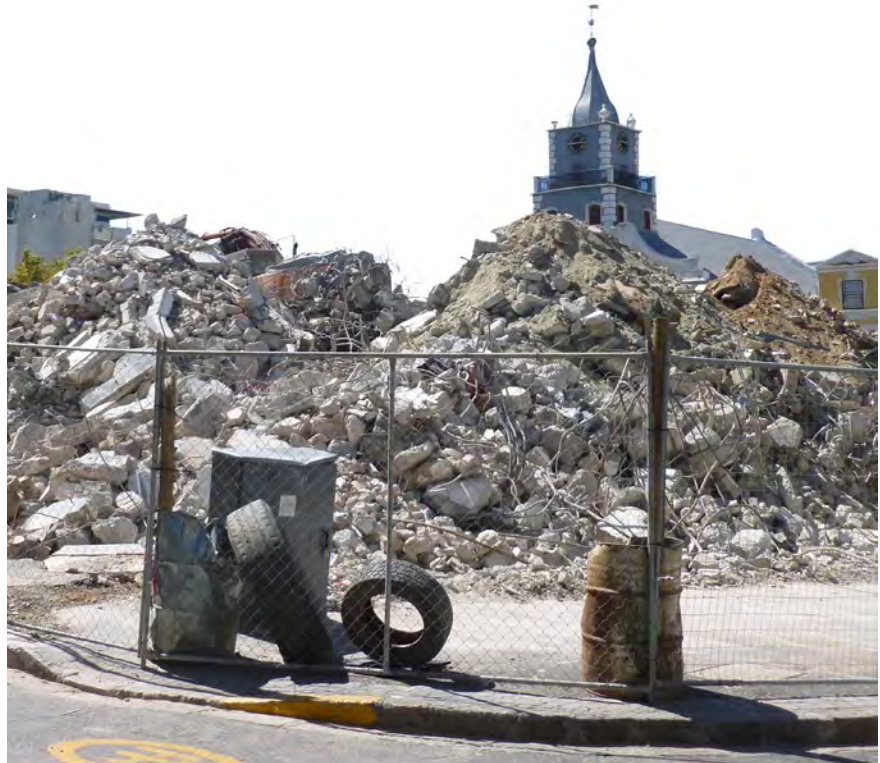
Figure 29: The recently demolished Tulip Hotel rubble. A new hotel shall be erected in its place.
