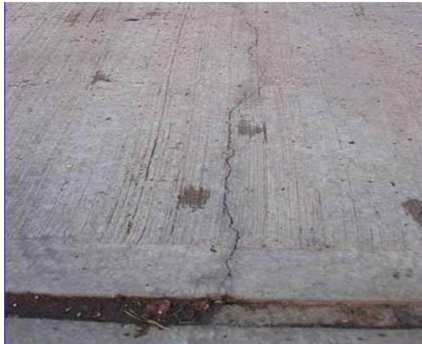
Figure 3. 4: Drying shrinkage cracking [41].
