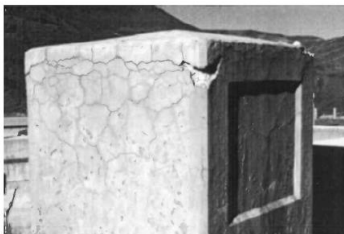
Figure 4. 4: Random cracking in a parapet wall caused by ASR [76].
