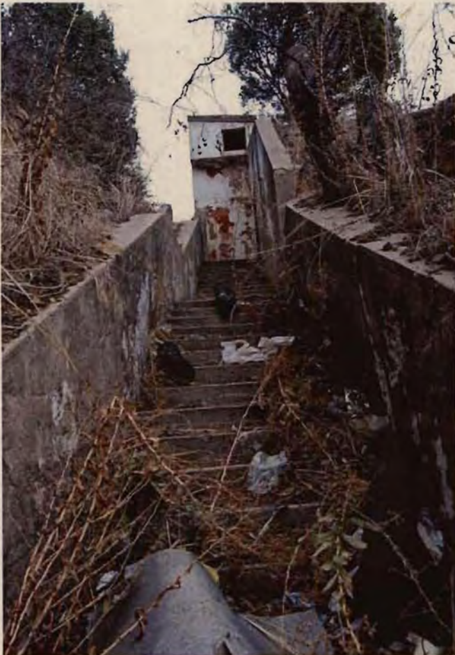
Figure 33. Nature reclaiming the concrete.
