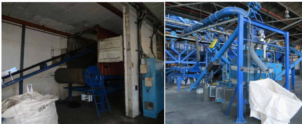
Figure 2.12: Tyre recycler factory at Atlantis
