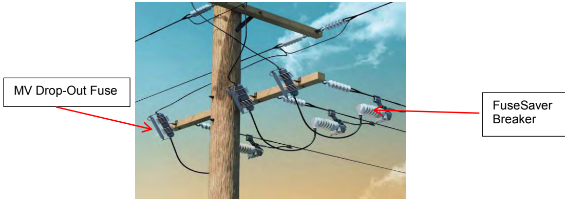
Figure 4.19: FuseSaver breaker protecting the Medium Voltage Fuse from Transient Faults [19]
