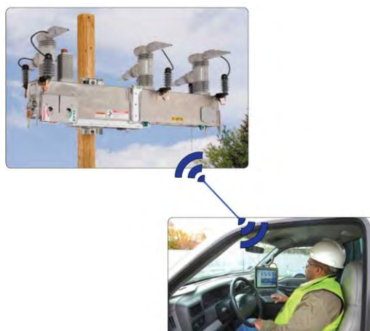
Figure 7.6: IntelliRupter control and communication module is configured and operated using a secure WiFi communication link [9]
