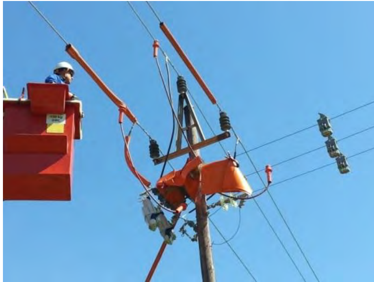
Figure 1: Overhead crew members from Eskom Western Cape Operating Unit distribution, install a Tripsaver Dropout Recloser as part of the pilot project – Waterkloof F1 11 kV Feeder
