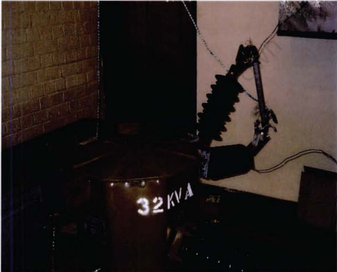
Figure 4.4 This photograph shows the fuse link which, for stability purposes, is mounted on the 32kVA SWER transformer. The MV output is connected to the base of the fuse link. The top of the link is connected via cable to the electrode (the cable is shown at the top of the photograph). The fuse has fallen, closing the link, resulting in a fault. The nylon rope used to raise and drop the fuse is seen connected to the fuse.
