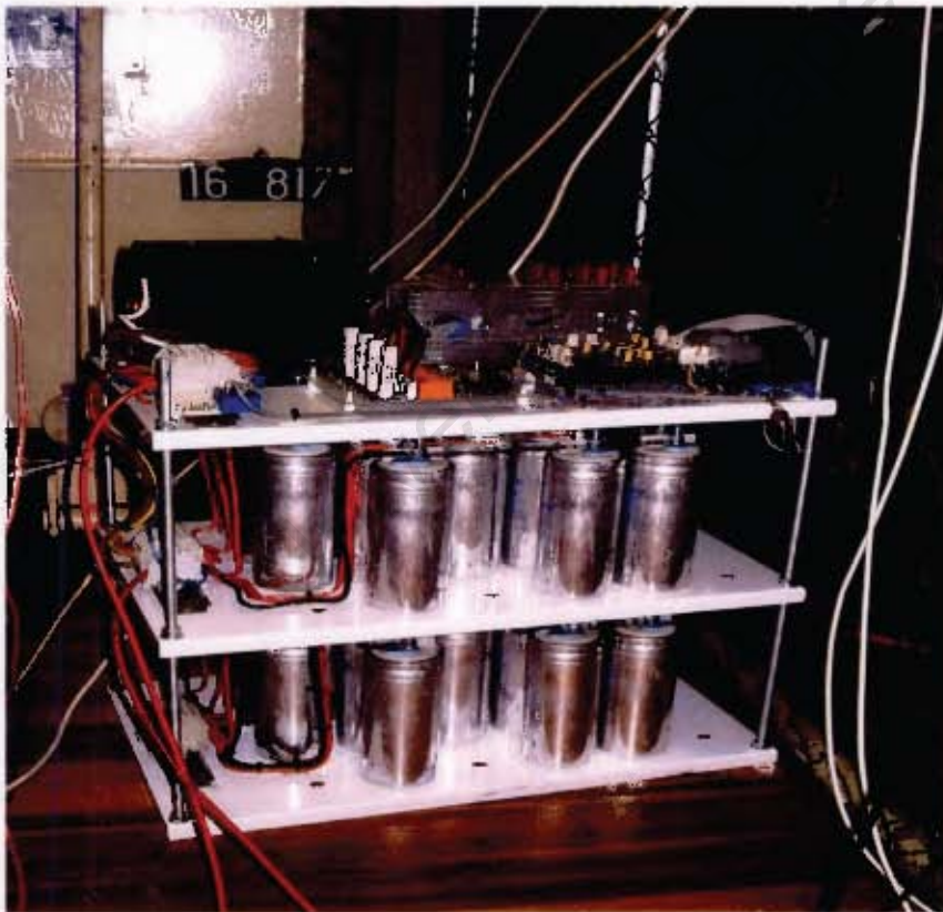
Figure 4.13 This photograph shows the compensator. The 50 \mu F capacitors can be seen on the bottom two levels, while the power electronics can be seen on the top of the compensator.
