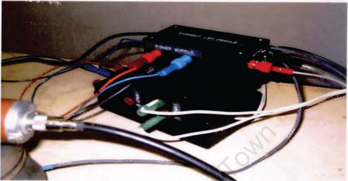
Figure 4.18 This photograph shows the current LEM, the voltage Differential Probe, and the power supply which powers both of them.
