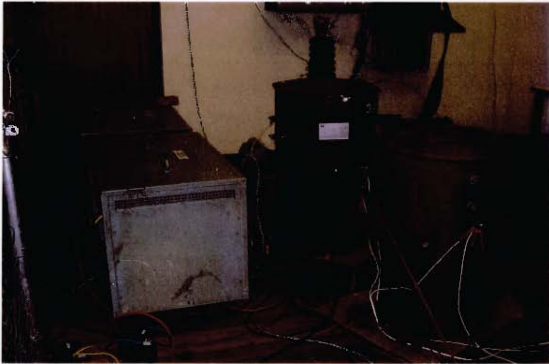
Figure 4.2 This photograph shows the two 48kVA transformers (T2 and T3) to the left (the two grey box-shaped transformers), the 32kVA SWER transformer (T4) to the back right, and the 16kVA SWER transformer (T5) to the front right.
