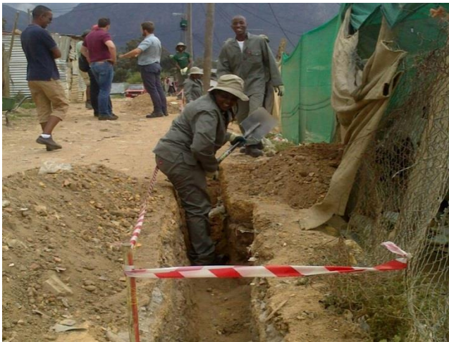
Figure 5.7 The community of Langrug digging trenches for pipework in connecting to greywater disposal pits, courtesy: GOS, 2016
