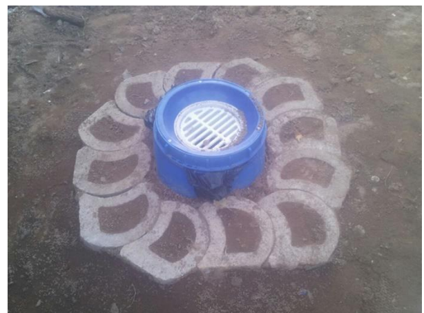
Figure 5.4 An example of a co-created greywater disposal unit developed by GOS, courtesy: GOS, 2016
