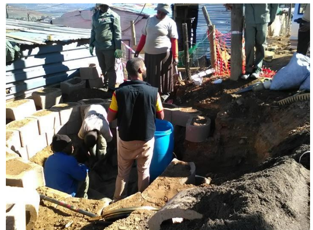
Figure 5.16 Community members constructing a tree pit in Block S in Langrug, courtesy: GOS, 2016
