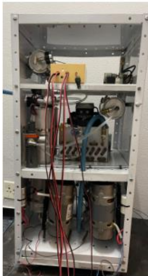
System Connected to control panel Circuit board and a power supply
