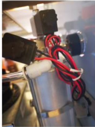
Connected 12v DC Solenoid Valves and Pneumatic Gauges on the Outlet of the Sieve Bed
