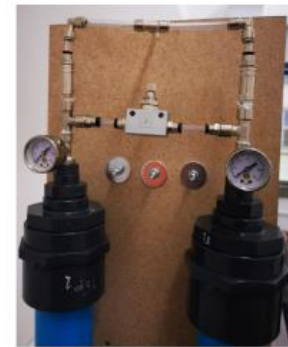
Top part of the Sieve Beds fitted with Pressure gauges and an equalization control valve. Both Sievebeds are connected to the product tank via non return valve
