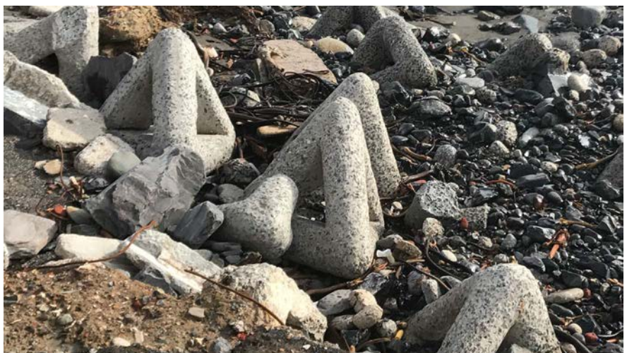
Fig. 23. Debris on the shores in front of the wall, a place where boulders and concrete is reduced to smooth stones and sand. The beach is also littered with tangled and rusted steel from the reinforcing of broken dolos.
