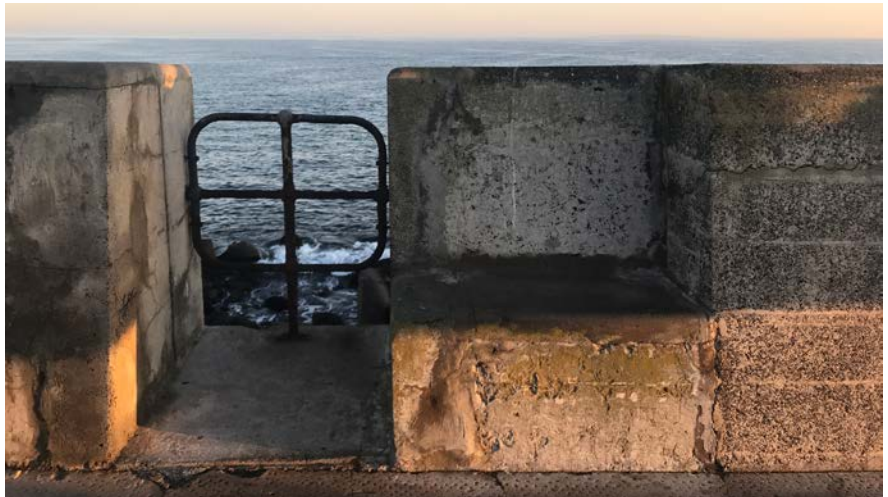
Fig. 21. Rusted balustrade set into the old breakwater wall.
