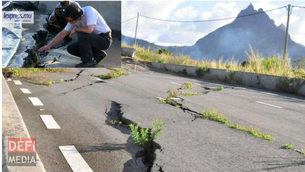
Figure 6-1: Possible settlement failure of Terre-Rouge-Verdun Road, Mauritius (L'express, 2015, Defimedia.info, 2016).
