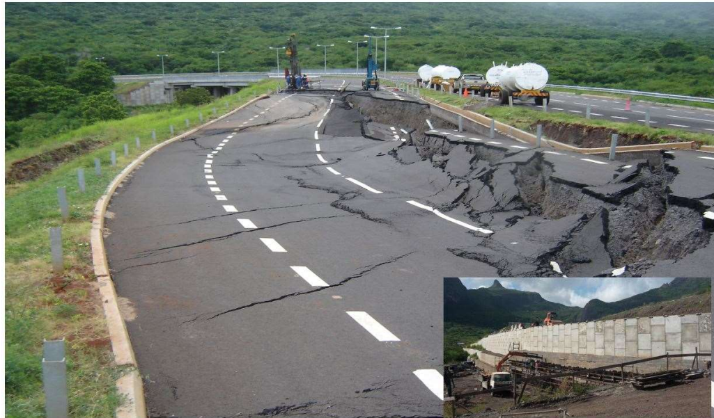
Figure 2-7: Ring Road, Mauritius. The bottom right picture shows the construction of the MSEW (ARQ, 2014).
