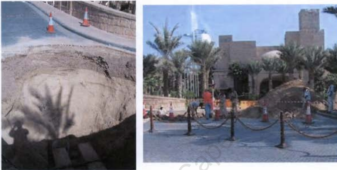
FIGURES 1.7 & 1.8: Damage caused to the road from pipe failure [7]
