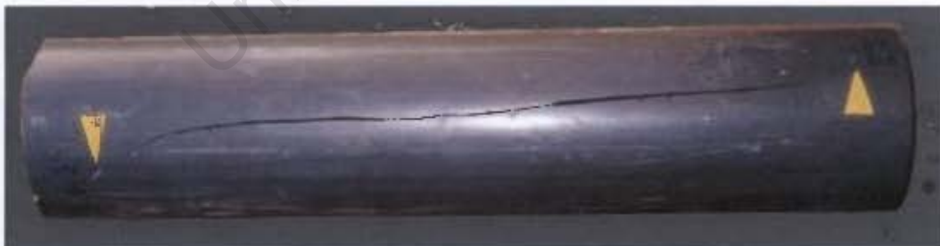
FIGURE 1.6: Example of pipe failure from the resort [7]
