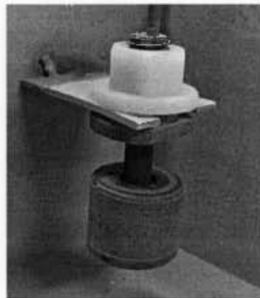
FIGURE 3.13: Float switch installed in the bath
