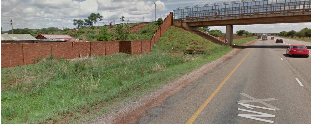
Figure 2.6 Brick Wall Self Enforcing Feature at Mookgophong , N1 in Limpopo Source: Google Earth, 2017
